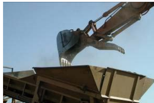
Loading urban wood waste into a screen hopper; Carson City, NV. Source: USDA Forest Service
