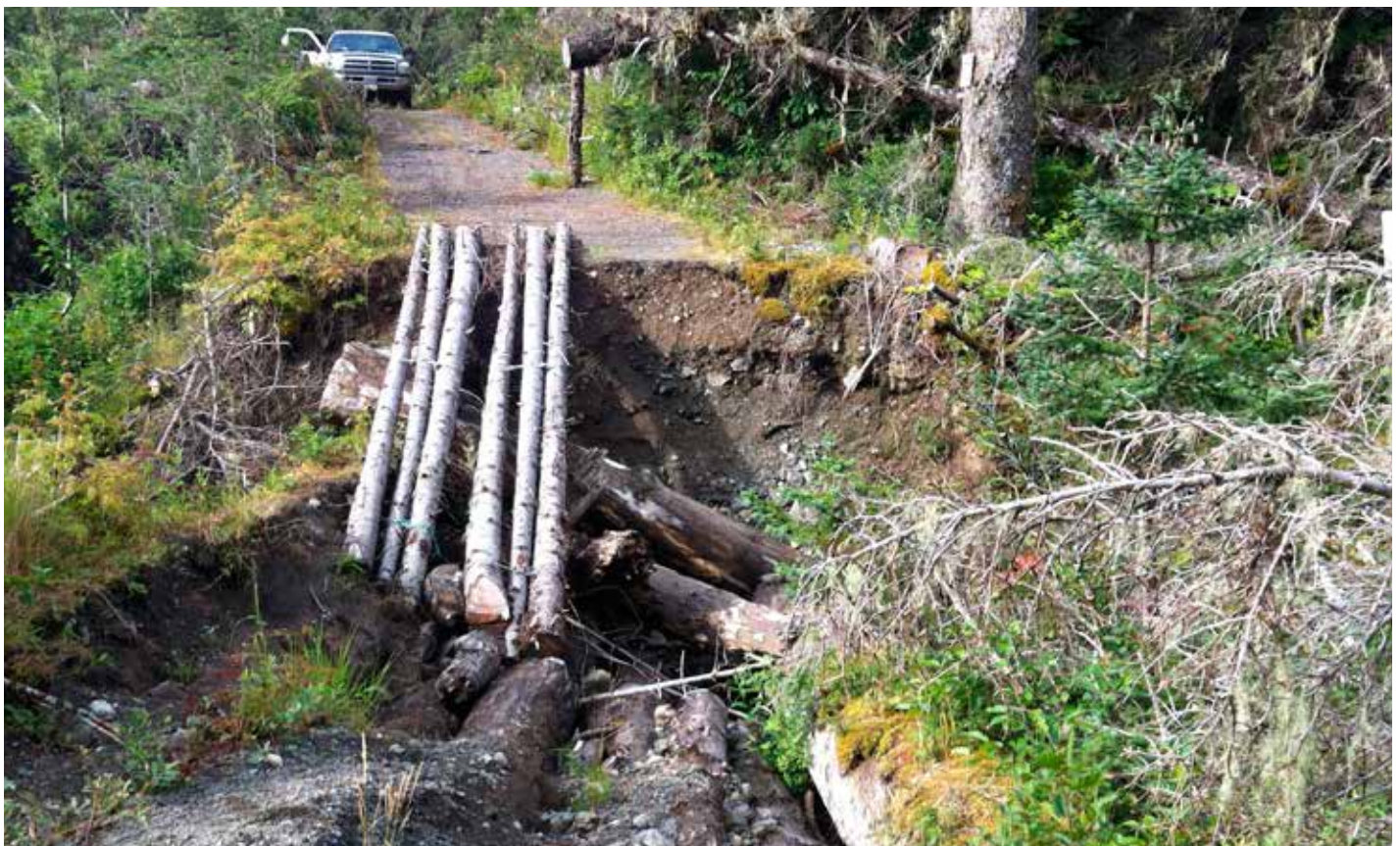
Collapsed stringer bridge, Chugach Alaska Native Corporation, southcentral Alaska.
