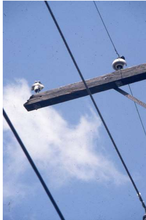
BROKEN CROSS-ARM INSULATOR
