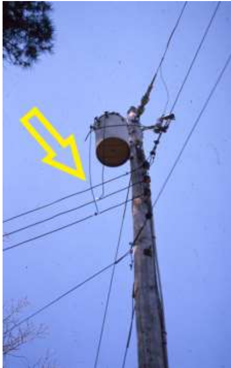
ARCING WIRE at TRANSFORMER
